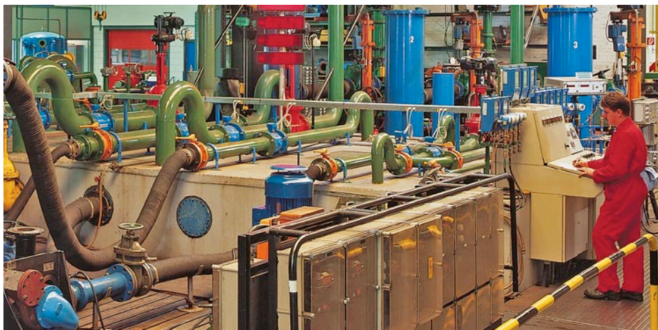
Proefstand SPX Process Equipment NL in Assen
